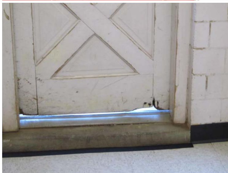
Gaps at the common door threshold at Building 1728
