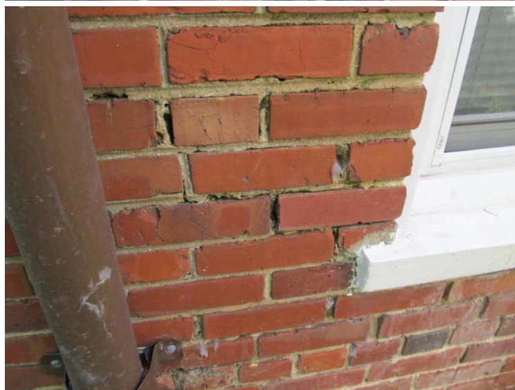
Mortar loss and deterioration at 1742 N. Rhodes Street
