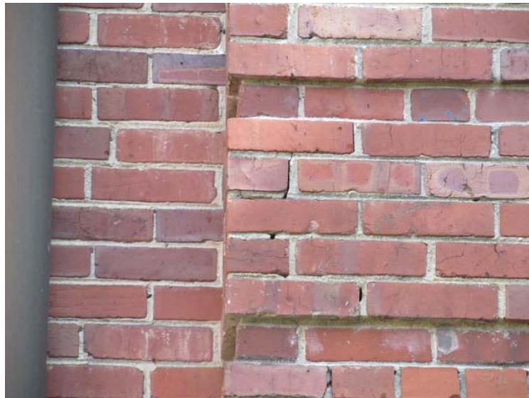
Mortar loss and deterioration at 1853 N. Rhodes Street
