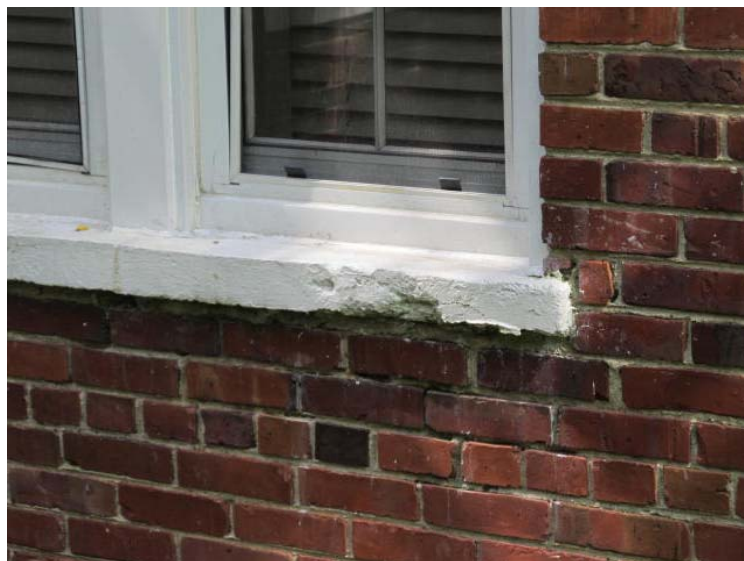
Sill deterioration at 1742 N. Rhodes Street
