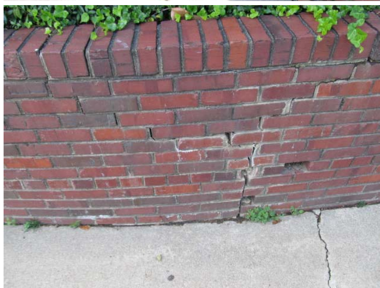
Retaining wall cracks and deterioration
