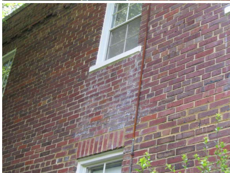
More significant efflorescence at 1739 N. Troy Street
