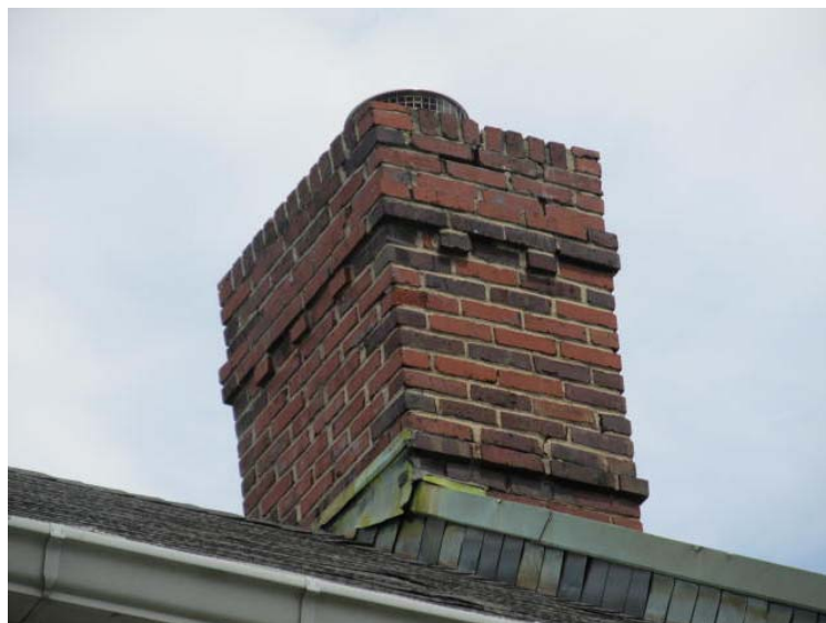
Chimney in need of rebuilding at Building 1782 North Troy Street
