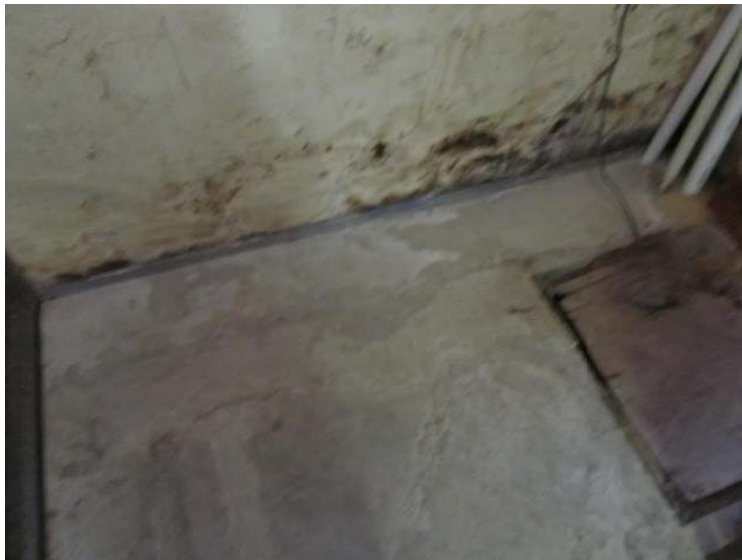
Evidence of past water infiltration at basement
