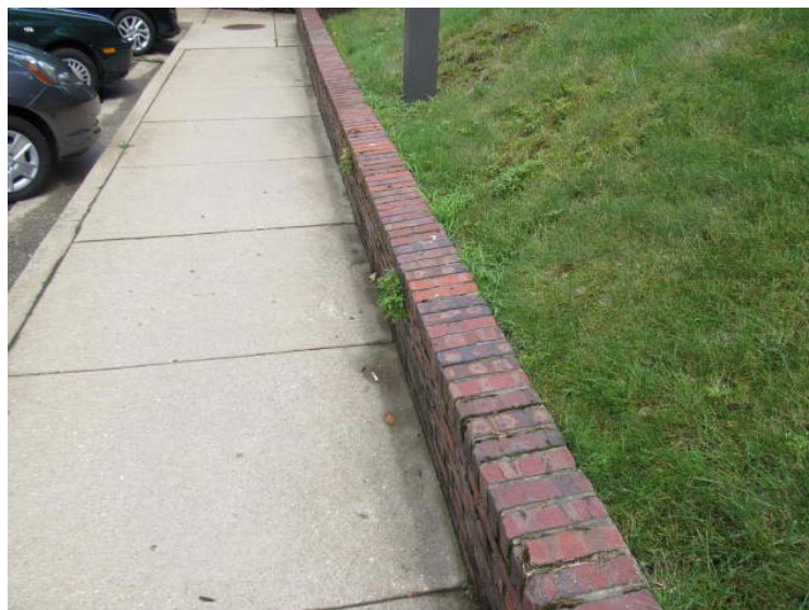
Slight retaining wall lean
