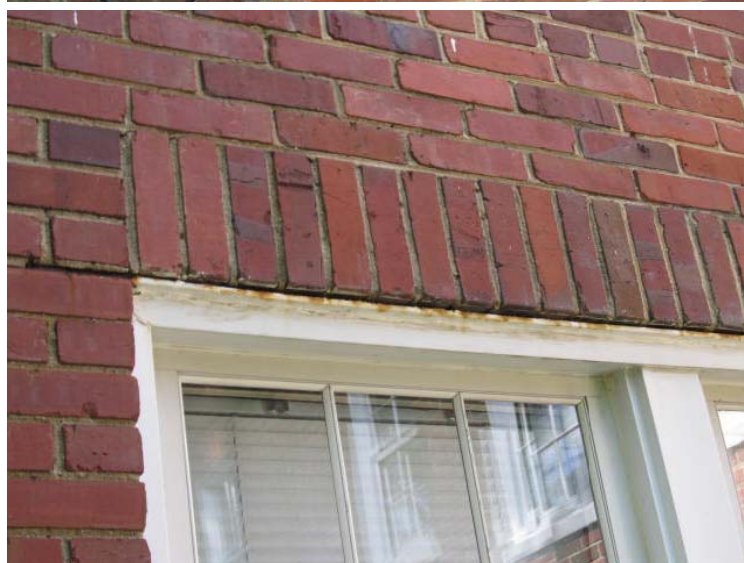
Metal lintel deflection and rust at N. Rhodes Street
