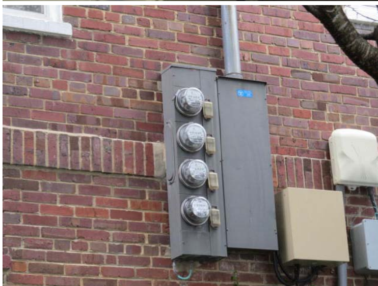
Electric meter panel
