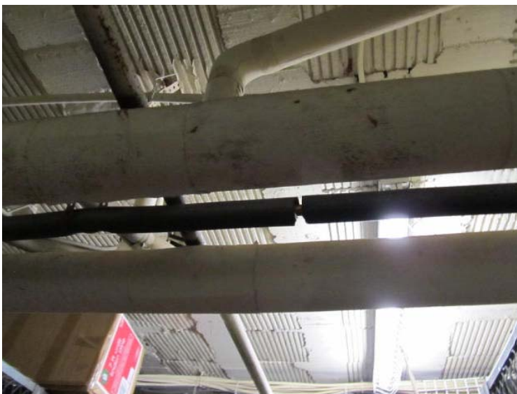
Domestic water pipes
