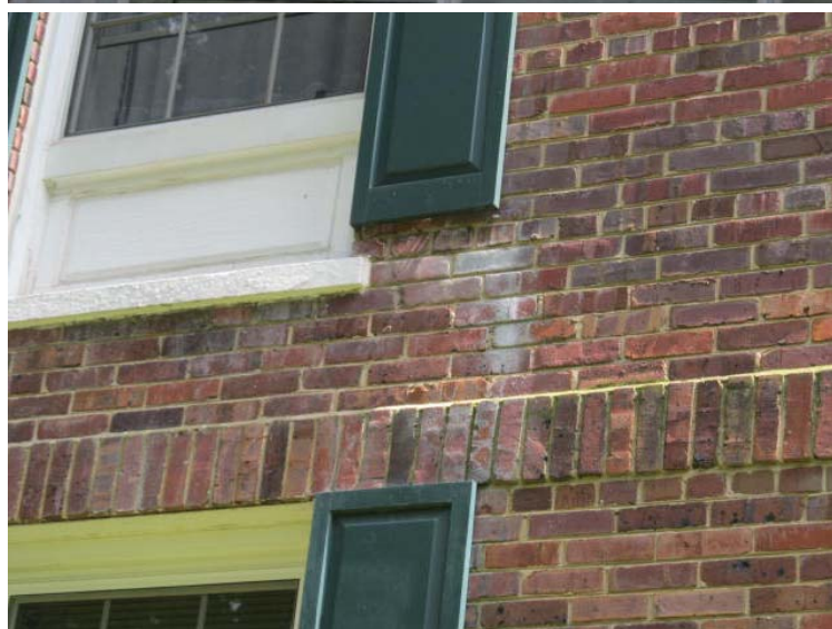
Minor efflorescence at 1741 N. Troy Street
