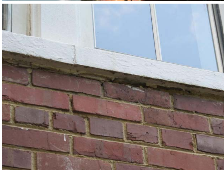
Mortar deterioration below sill at 1758 N. Rhodes Street
