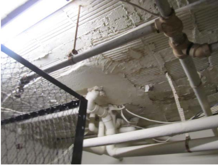
Domestic water pipes
