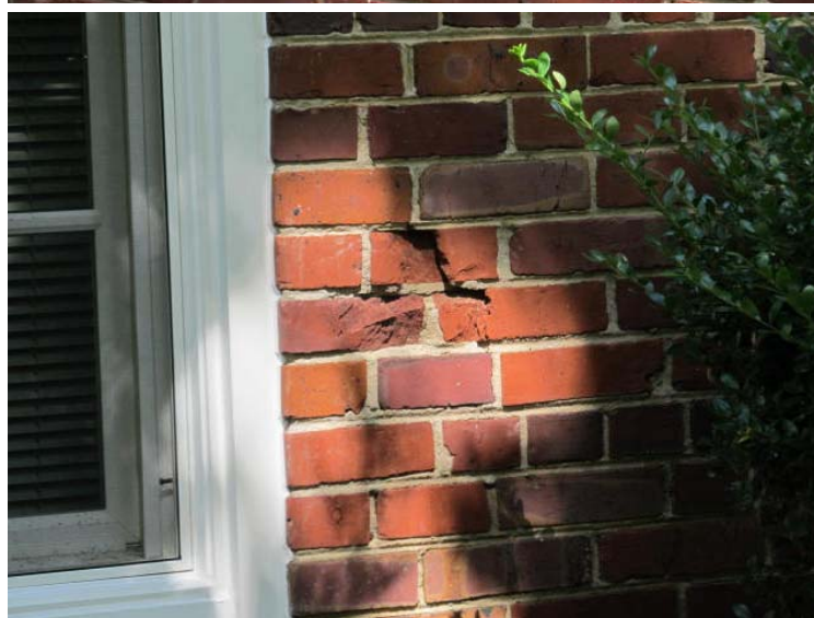
Brick spall at 1744 N. Rhodes Street
