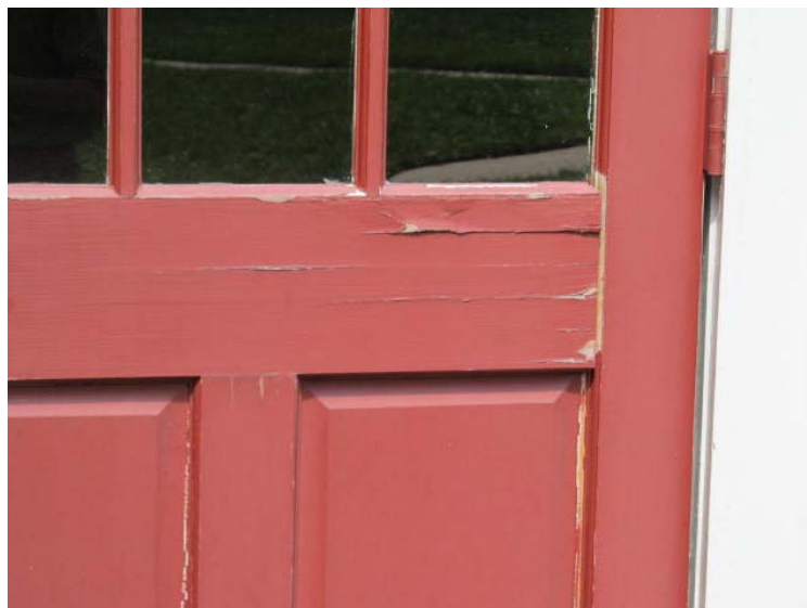
Significant deterioration of the door at Building 739
