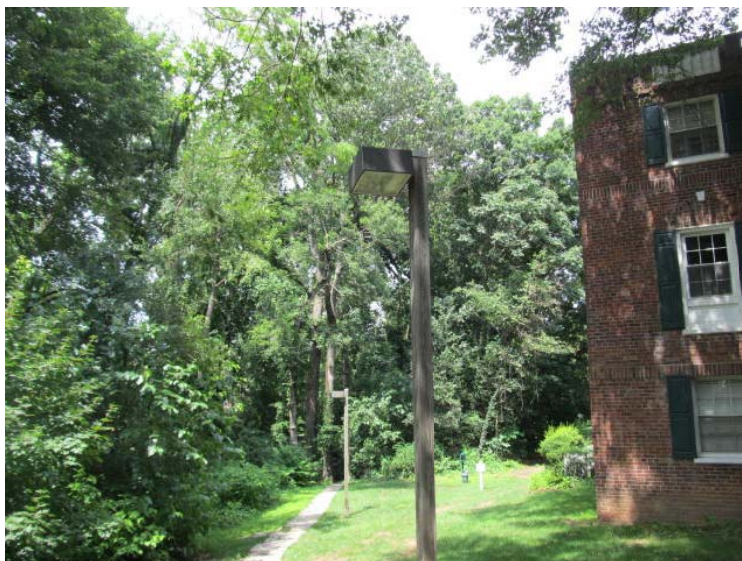
Light pole and fixture
