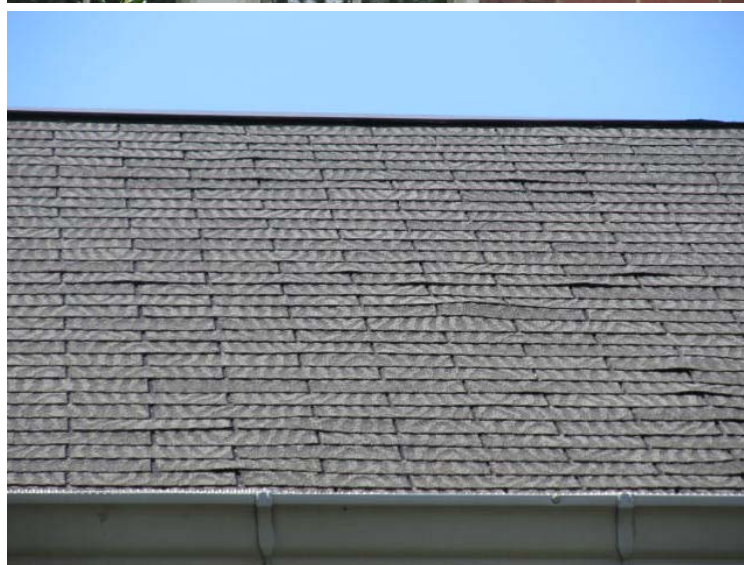
Typical asphalt shingle lift and deterioration
