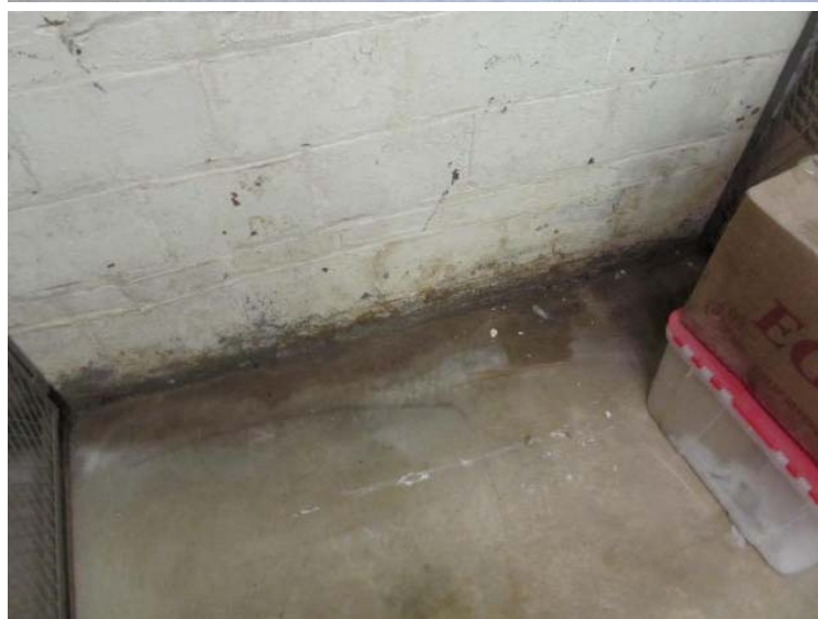
Active water infiltration at basement
