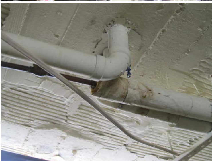
Discolored insulation at pipes is early indication of leak
