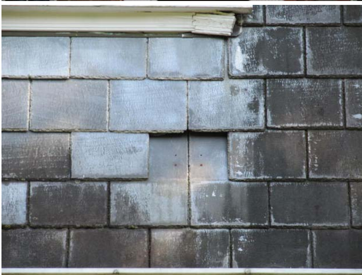
Missing synthetic slate shingle at Building 1806
