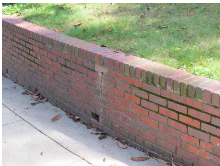
Retaining wall cracks and deterioration
