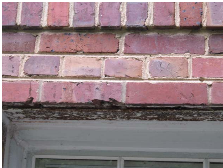
Lintel rust and minor brick spall at 1782 N. Troy Street
